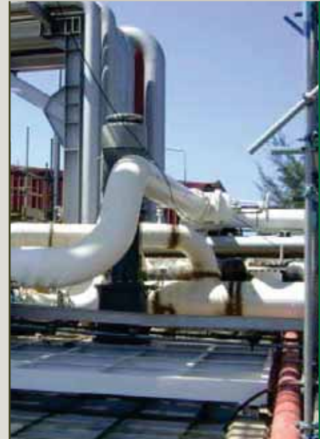
Piping systems at the Miri Crude Oil Terminal in Miri
